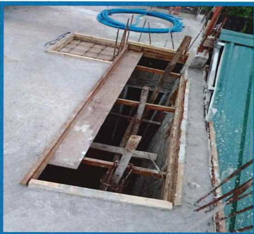
This will be the second floor where my family will stay. That is the stairway.
