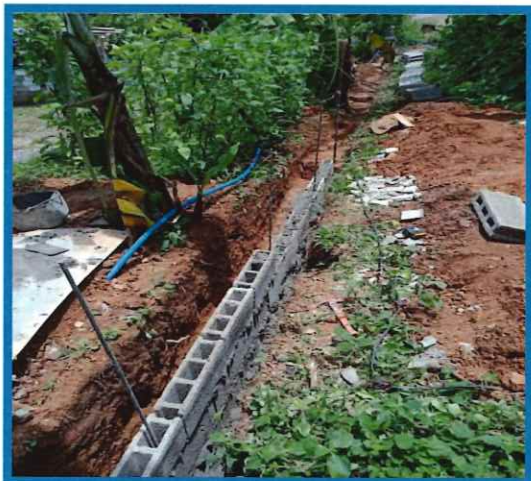
This is the water-way to avoid flooding in our place.
